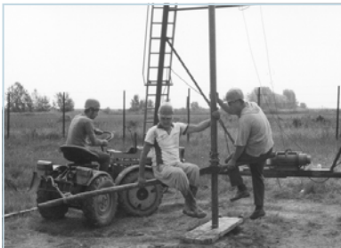
Excavators use simple tools to extract the mud from the reserve area in Hungary
